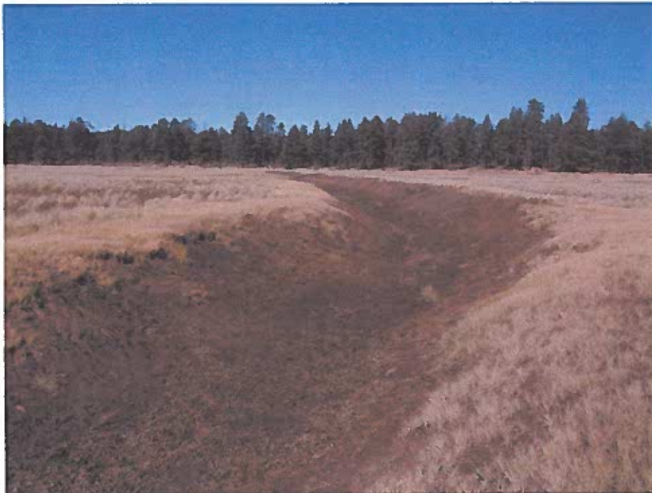
Figure 4. Allan Lake excavated channel. Note the lack of moisture and vegetation in the channel sides & bottom. Photo taken in November 2004 (NCD).
